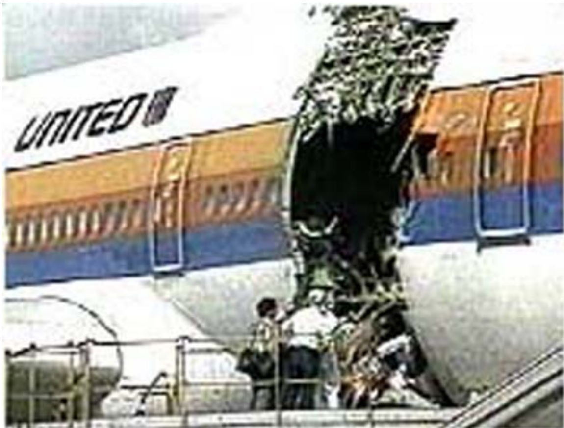
Caption for above photograph: Photo of hole in United Airlines Flight 811 made by inadvertent opening of forward cargo door in flight.
